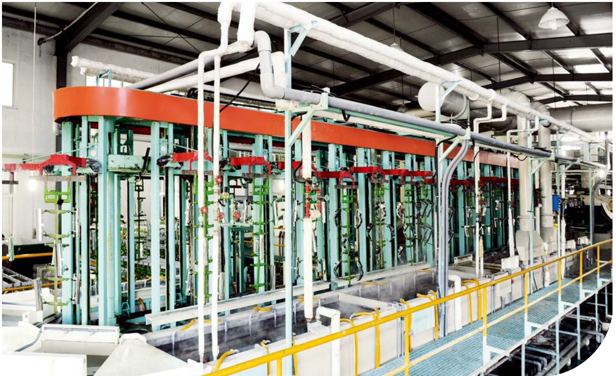
Automatic plating lines to ensure the stability of the highest quality product finishes that can never be achieved using manual methods.
